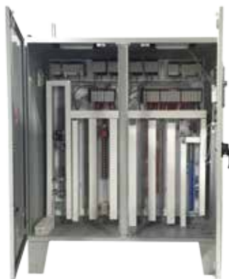
BMS and Control Panels
